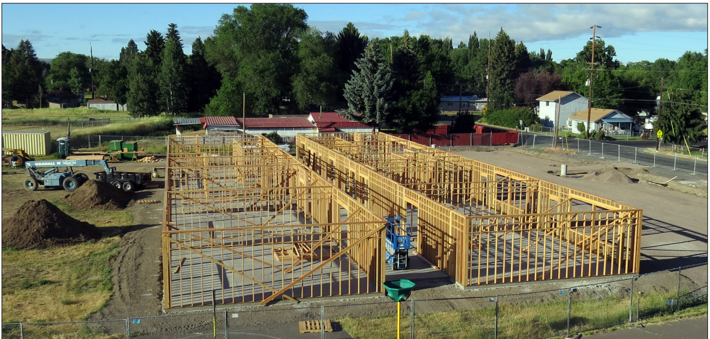
Construction on the new classroom building at Stearns Elementary School began in March 2020. The new addition will have eight classrooms, including four for the district's special services programs. The project is expected to be ready for students in early 2021.
